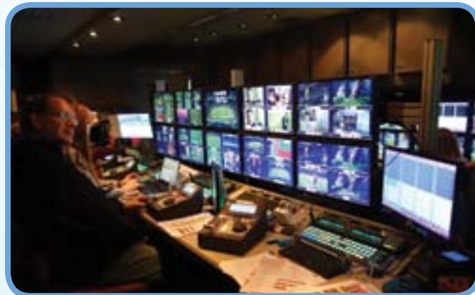
Sports Venue Control Room Operations
